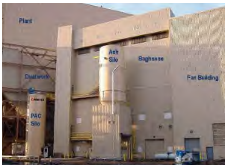
TOXECON™ System Installed at PIPP
